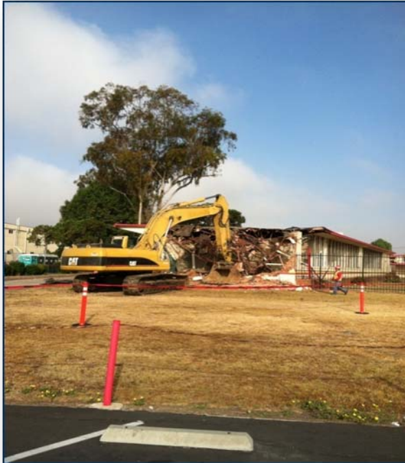
The full removal of building #4 to make way for a new access road for the campus.
