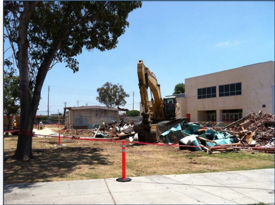
Demolition of multiple buildings this Summer to make way for Phase 1A.
